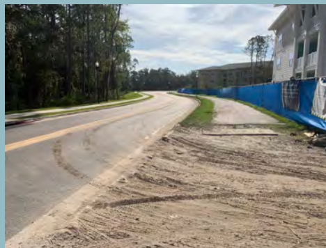
Sediment tracking from a nearby construction site
