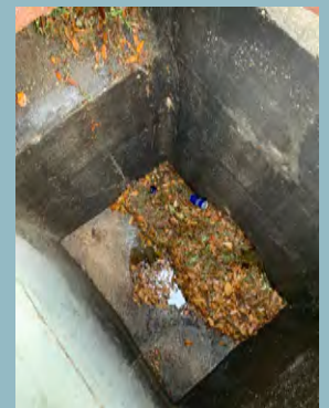
Resident blowing yard debris down a storm drain
